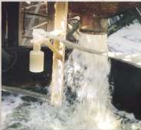
KAB 10 Transducer together with the SUMPI is being used to measure level in a water tank.
